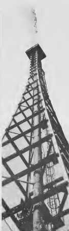
ALKY-2 FLARE is the refinery structural giant, standing well over 200-foot high.
